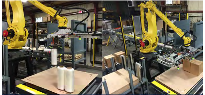
The same robot palletizing both cases and rolls as they come in from different infeed conveyors.
