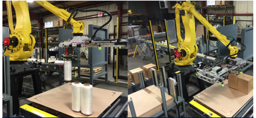
The same robot palletizing both cases and rolls as they come in from different infeed conveyors.
